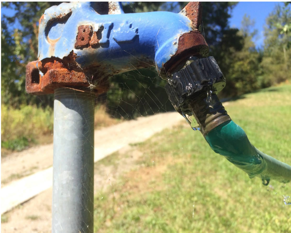
Figure 12 - One of the dozens of leaking faucets encountered by the Ambassador
